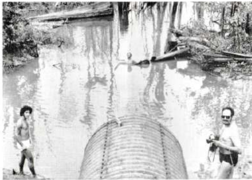
The huge (six feet in diameter) corrugated drain has formed a "flood pool" by the erosive action of the quickly moving water.
